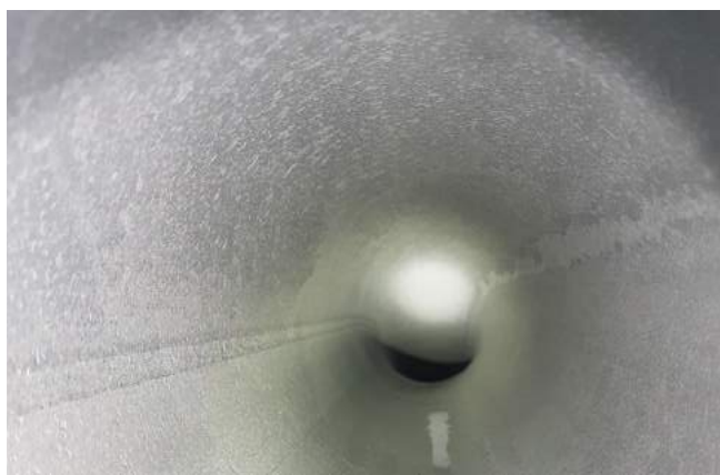
Figure 2. A pipeline after EnerClear Services' in situ mechanical and chemical cleaning process.
