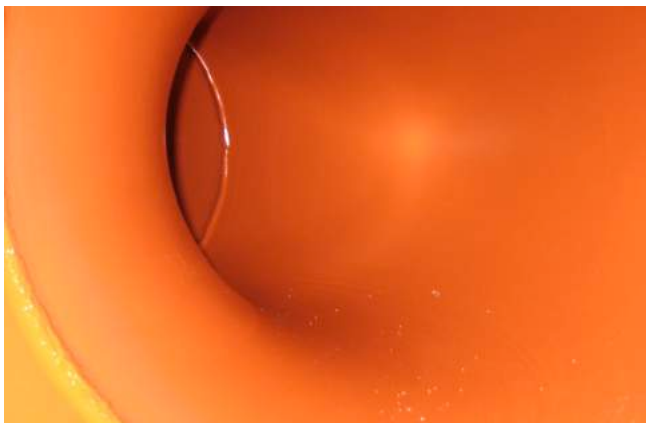
Figure 5. In situ coating provides full homogenous coverage throughout the entire line, including all bends (ie: 45s and 90s), providing a solution for pipe racks and difficult to access lines.
