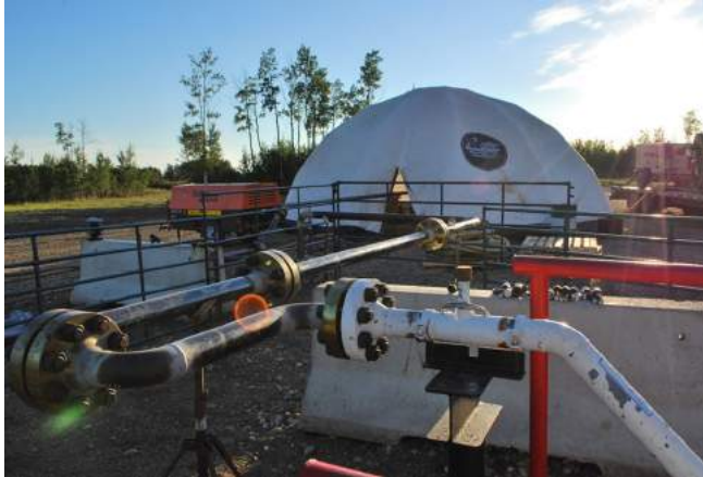
Figure 3. A typical EnerClear Services set-up. Footprint shows launcher/receiver tent with temporary pipefitting (20 - 25 ft run-out spools) extending out (to 90°) to a convenient location.
